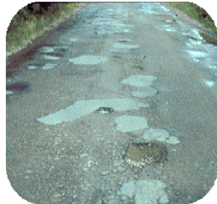
Roads and structures constructed in filled wetlands often suffer subsidence
