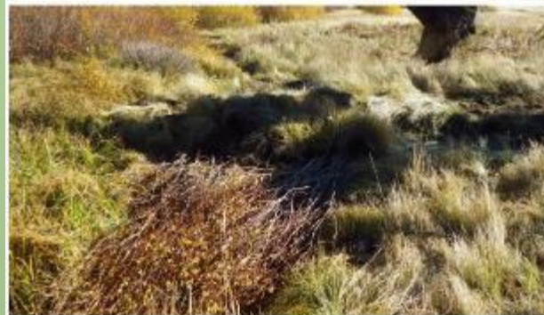
7. Final sod lift being installed over third brush lift. Each dam typically included 4 layers of sod and 3 layers of brush.
