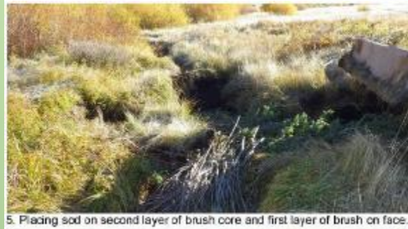
5. Placing sod on second layer of brush core and first layer of brush on face.
