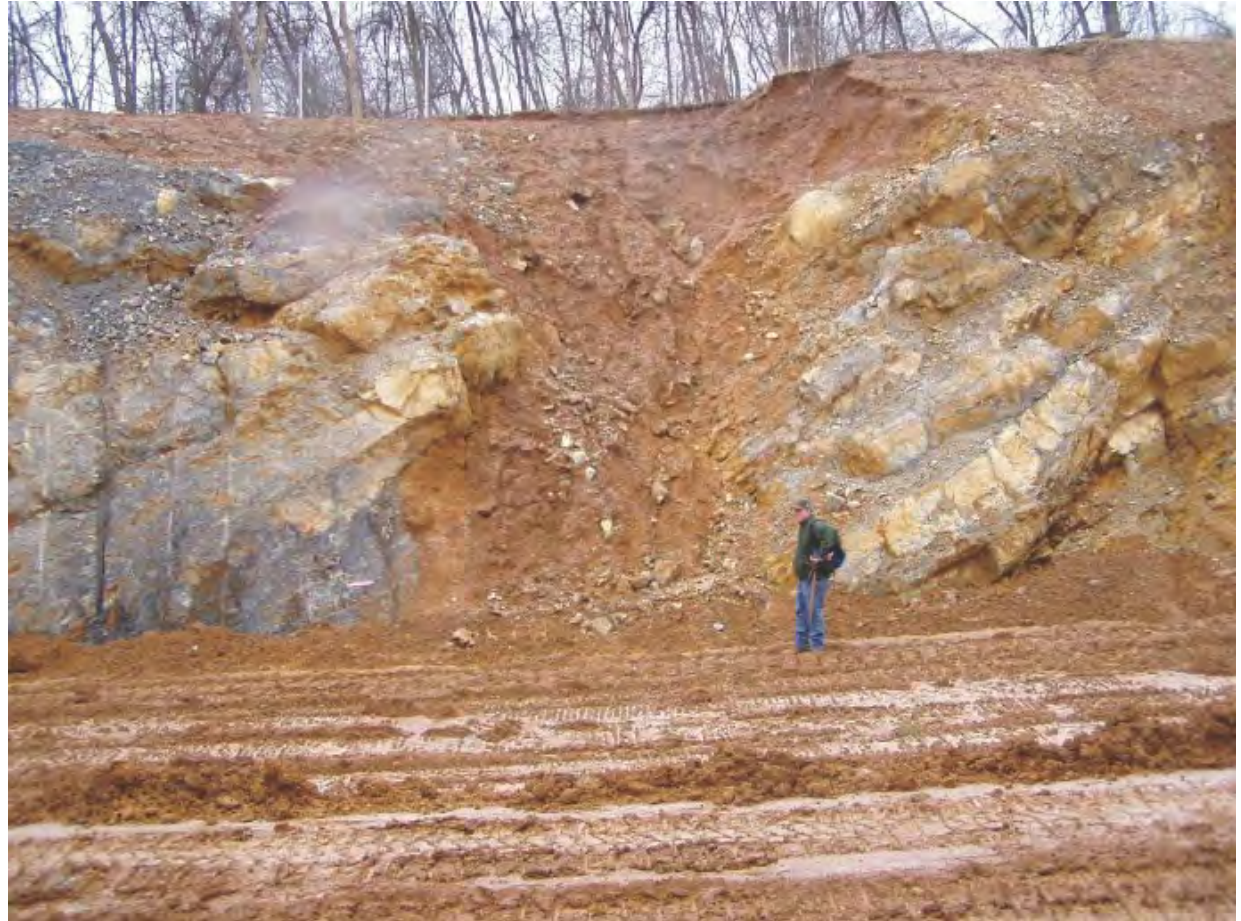
Filled solution joint/sinkhole
