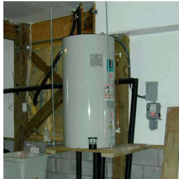
Figure 31: Example of Elevated Utilities
