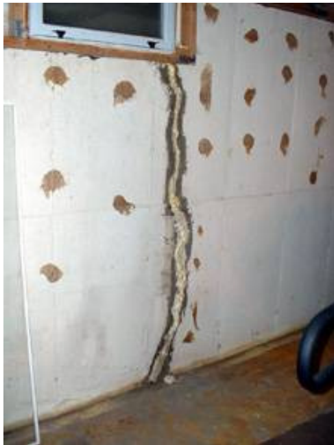
Cracked basement wall in Amherst, New York area.
