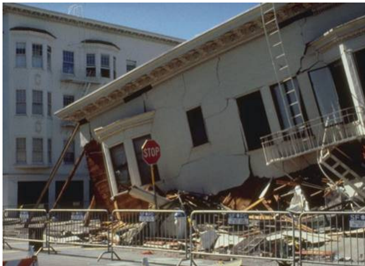
Earthquake damage from the Loma Pieta earthquake of 1989 for an area of saturated fill in the Marina District of San Francisco. Source: New Geologic Maps Highlight Bay Area Earthquake Hazards; http://earthquake.usgs.gov/regional/nca/qmap/
