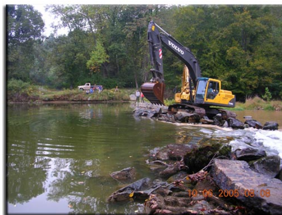
Restoration of impaired waters here dam removal is expensive and time consuming. Source: Maryland Department of Natural Resources
