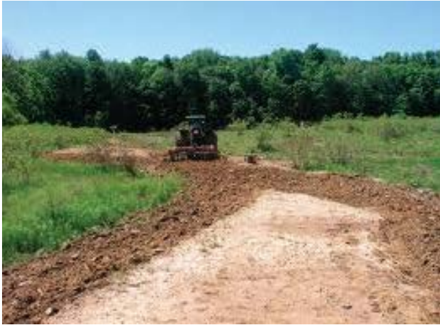
Crushing drain tiles. Lakes, streams, and estuaries often recover once chemical and nutrient pollution is stopped. However, active restoration such as crushing drain tiles is needed to address wetland drainage and fills and restore wetland hydrology. Source: Land and Water
