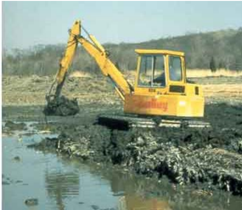
Fills in wetlands destroy natural flood storage and conveyance and all other wetland functions and values. Fills also commonly cause water pollution. Source: Fish and Wildlife Service
