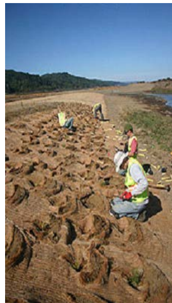
Active wetland restoration. such as revegetation is often necessary or advisable in cleared or excavated wetland areas where non-native or invasive species are believed to be capable of rapidly establishing and precluding establishment of native plant species. Source: Source: Giacomini Wetland Restoration Project, National Park Service
